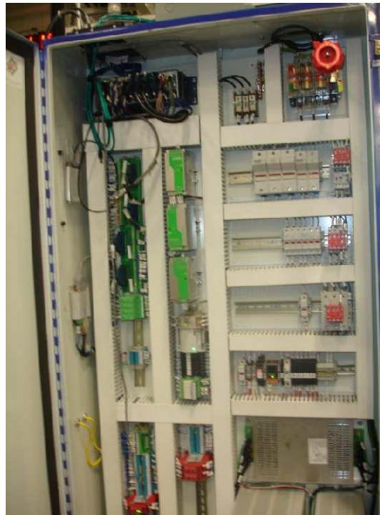
Figure 5: Main station panel
